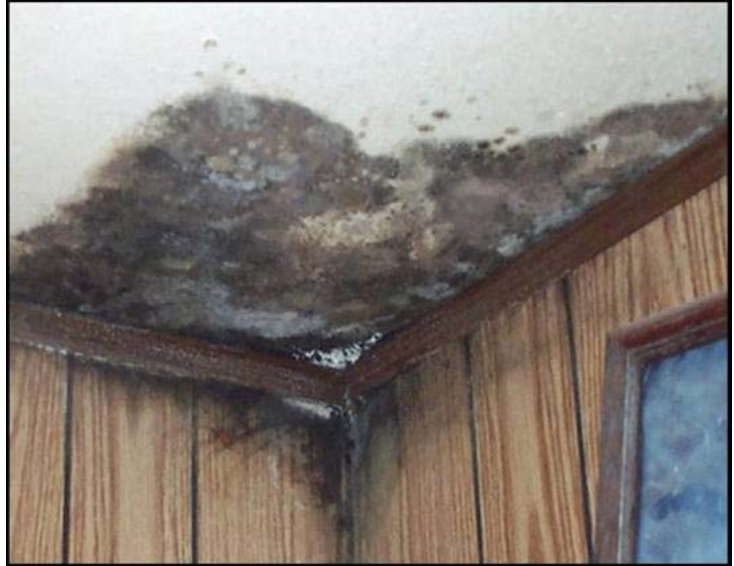
Mold caused by moisture in a home.
