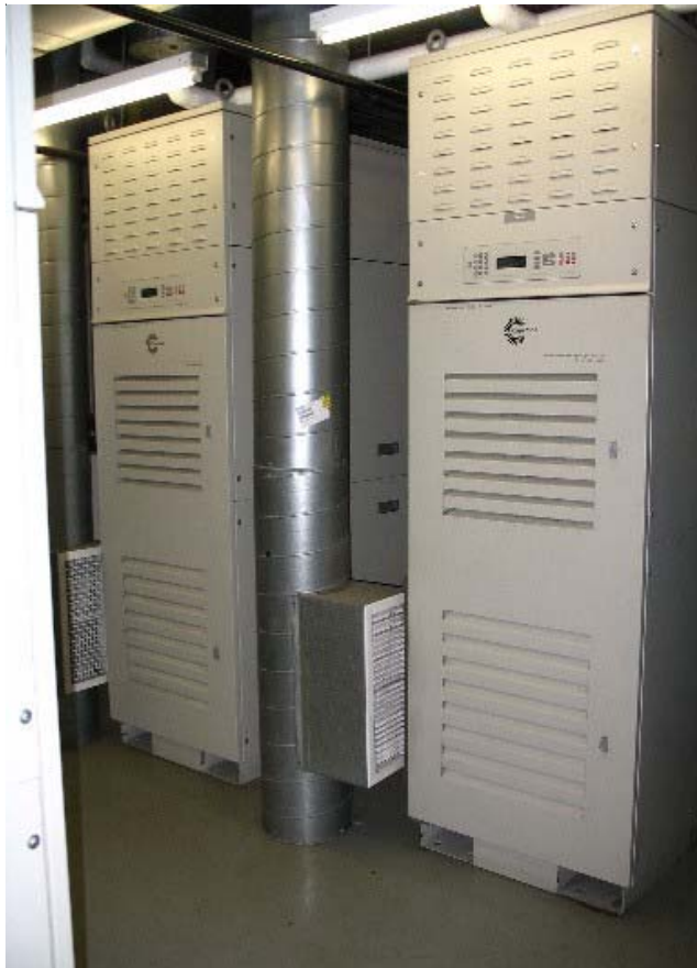
Two of TMA's four 60-kW microturbines
